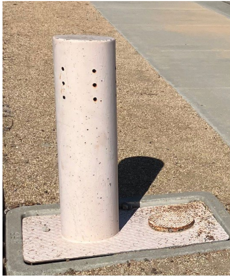
Figure 5. Typical Air Release/Air Vacuum Valve at Grade
