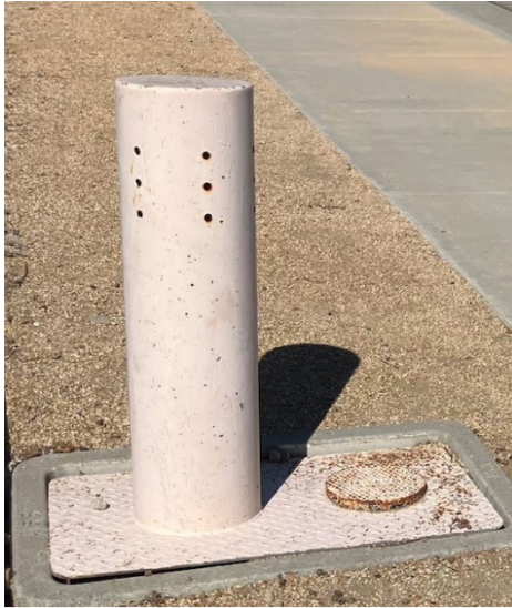
Figure 4. Typical Air Release/Air Vacuum Valve at Grade
